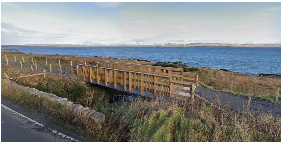
One of five bridges located along the Lochindaal Way. Image Capture: Dec 2021, © 2023 Google
